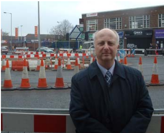
Cllr Brian Woodcraft surveys the ongoing improvement work at the Lee Green junction.
